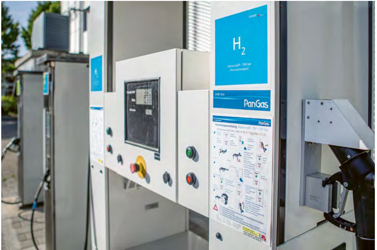
In move at Empa in Dübendorf, a hydrogen fueling station is in operation since 2015.
