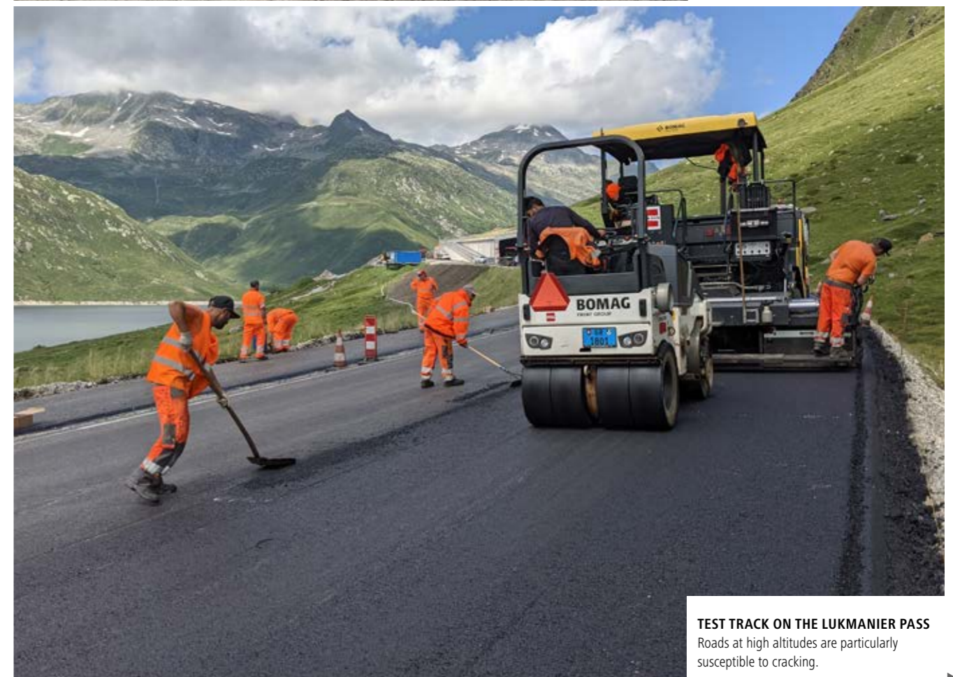
BLACK ASPHALT MOUNTAINS Swiss reclaimed asphalt should be returned to the roads as completely as possible.
