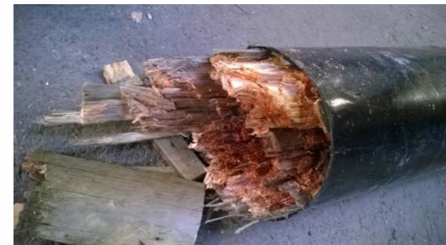
A wooden telephone pole felled by fungi. With the right non-toxic remedies, the poles’ lifespan can be extended significantly.
